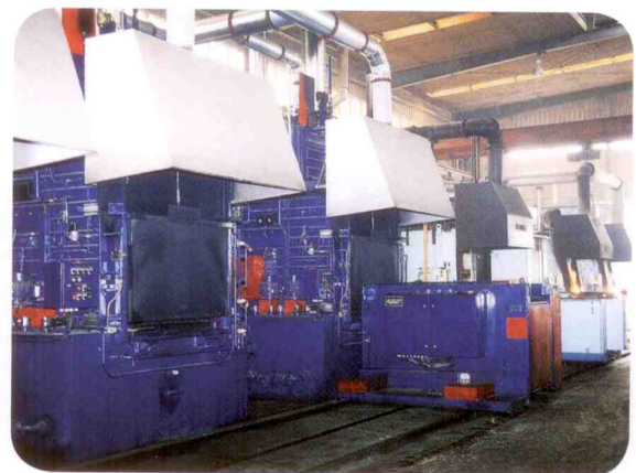
Furnaces for heat treatment process
