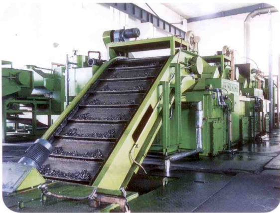
Conveyor furnace line used for roller and bushing heat treatment, e.g. carbon-nitriding
